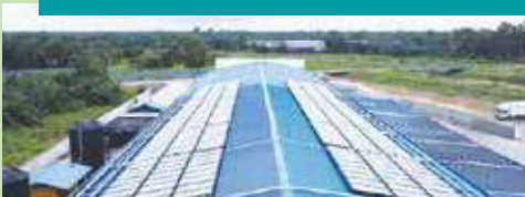
Solar thermal system installed at NB Poultry Processing Industries Sdn Bhd
