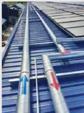
Hot and cold water piping
