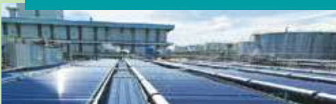
Solar thermal system installed at IOI Pan Century Oleochemicals Sdn Bhd
