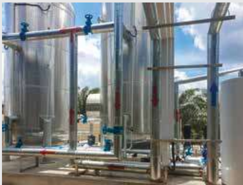
25,000L thermal storage tanks
