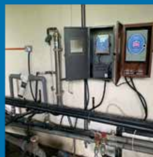
Electronic water conditioner at Cooling Tower 2
