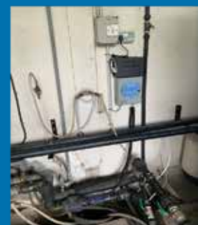
Electronic water conditioner at Chiller
