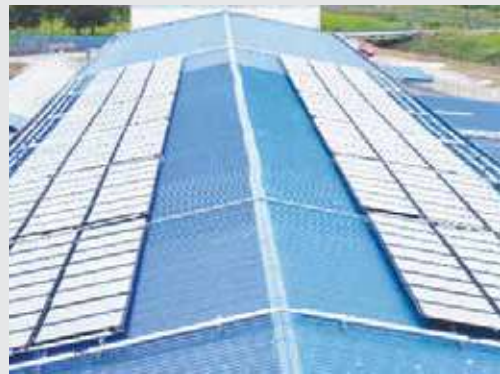
Solar collectors on rooftop
